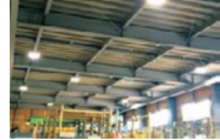
THK NIIGATA Distribution Center
