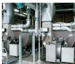
Vacuum hot water boilers
