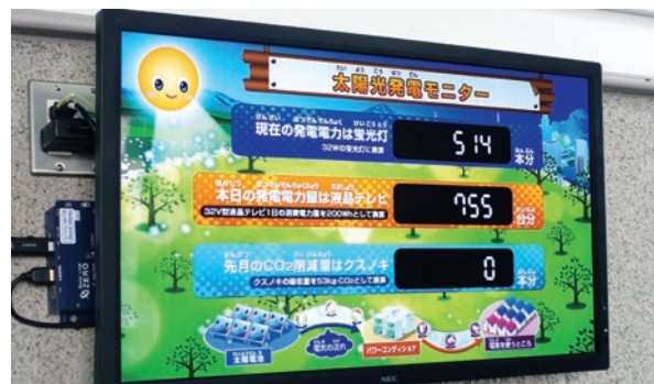
LCD monitor displayed in the lobby
