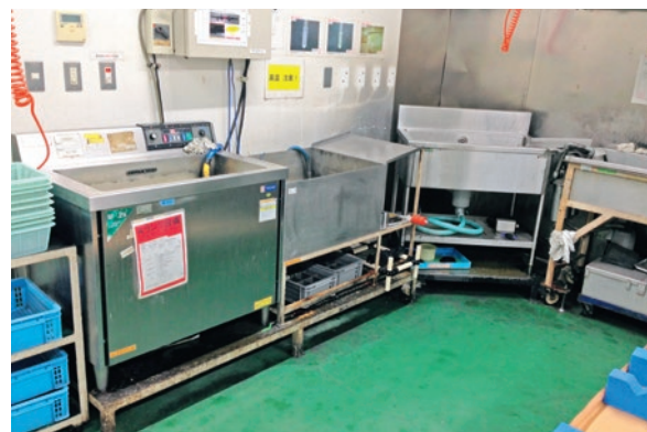
Washing process using new washing fluid
