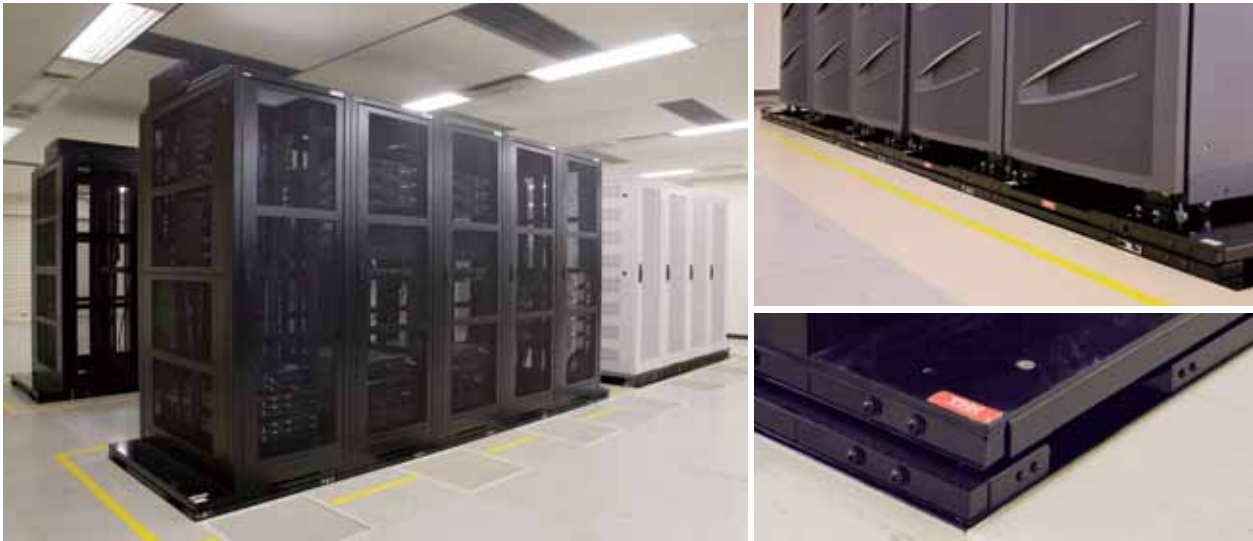
Seismically isolated JAL servers
