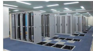
The entire transmission room floor is protected by seismic isolation devices.
