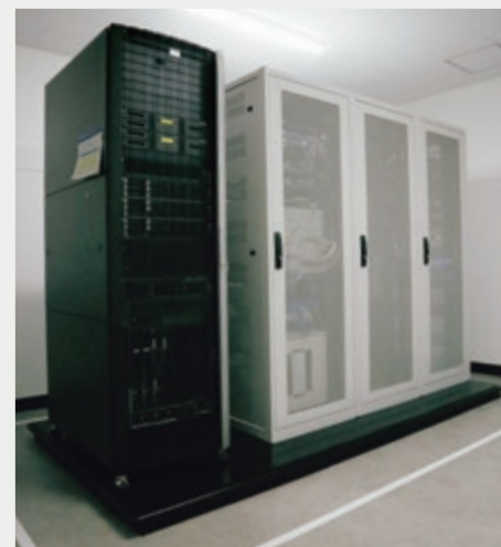
Servers in our new emergency shelter, safeguarded by seismic isolation
