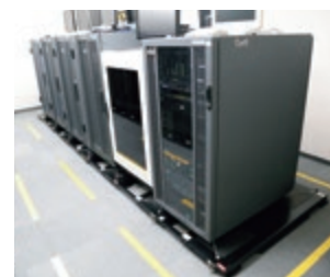
Servers with seismic isolation devices
