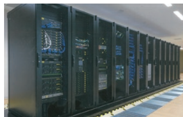
Servers with the Seismic Isolation Module Model TGS installed
