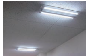
LED lighting in the corridor.
