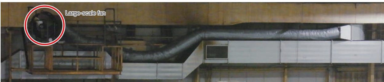
A large-scale fan directs recovered waste heat inside the plant.
