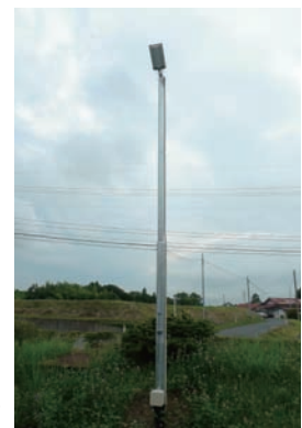
An LED light standard illuminates one of the plant's two parking lots.
