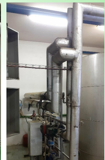
Compressor exhaust heat being utilized (TRA Czech)
