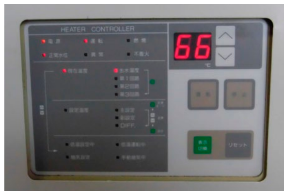
New digital control panel
