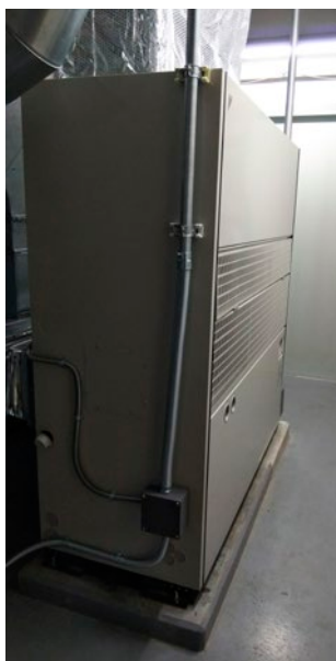
New HVAC unit for the precision measurement room
