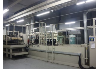
Newly installed semi-centralized coolant tank
