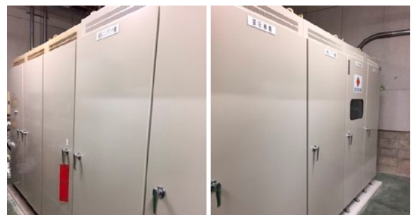
Electrical room with new transformer
