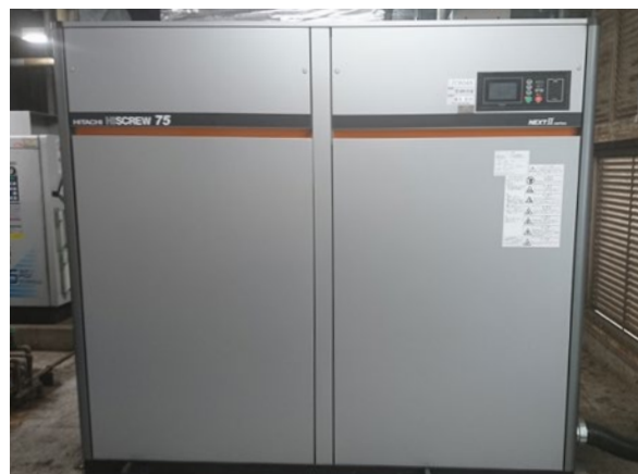
New air compressor in Factory 3
