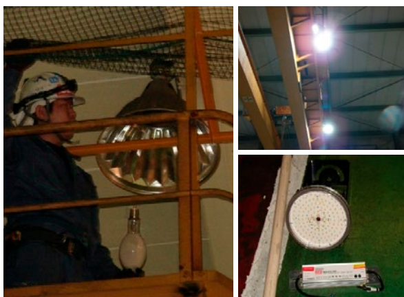
(Left) Removing mercury bulbs at the Sendai plant (Top right) Lighting after the LED upgrade (Bottom right) Newly installed LED light
