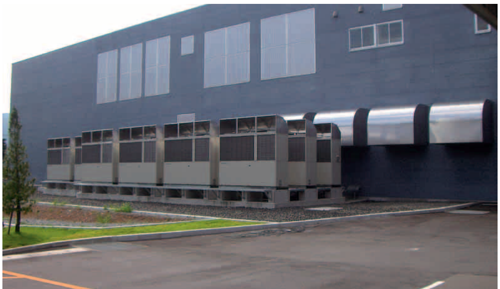
Gas-fired heat pumps that run on LNG (Chubu Distribution Center)
