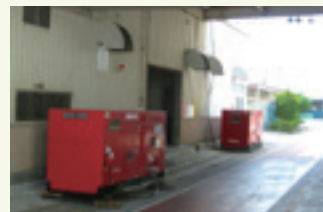
Generator introduced at the KOFU Plant
