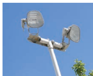
Parking lot light that is now set by a timer
