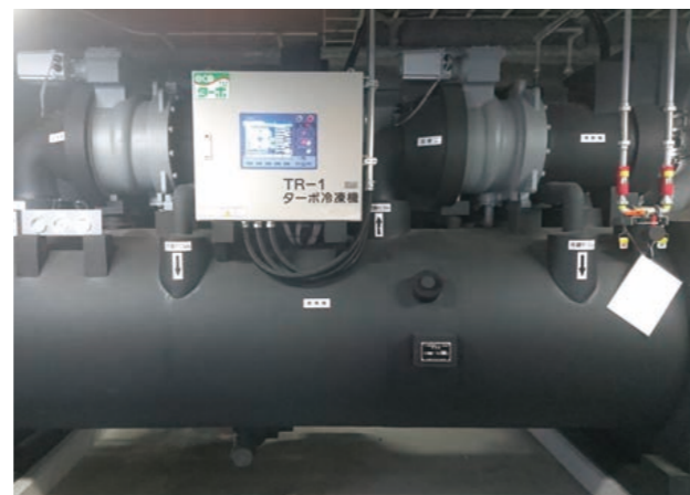
Newly installed inverter turbo chiller
