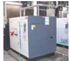
An air compressor at the YAMAGUCHI Plant
