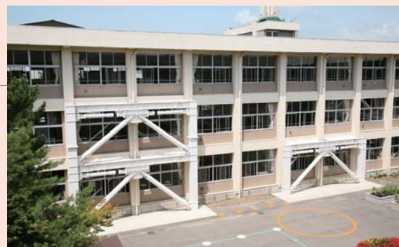
▲ Exterior of the Chikuzan elementary school building in the city of Akita after the installation of viscous dampers for quake-resistance
