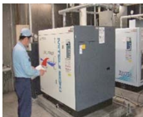
▲ Water-lubricated compressor at the YAMAGUCHI Plant
