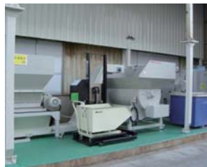
▲ Sludge solidification equipment at the KOFU Plant
