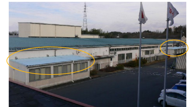
Quality Assurance Section office (left) and Manufacturing Section II production floor office (right) with coated roofs
