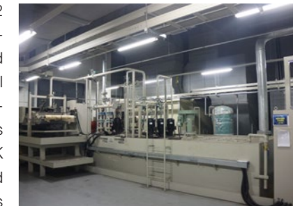
Newly installed semi-centralized coolant tank
