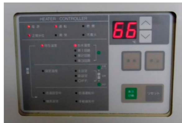
New digital control panel
