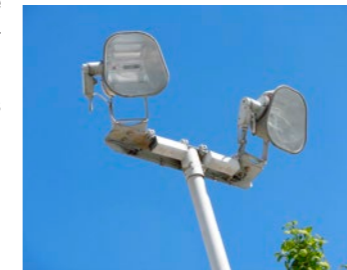
Parking lot light that is now set by a timer
