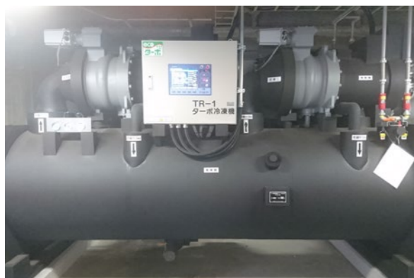
New inverter-type turbo chiller
