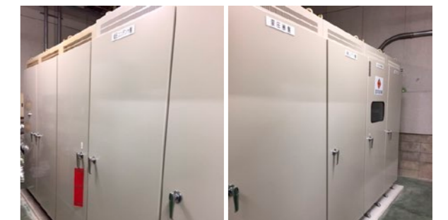
Electrical room with new transformer
