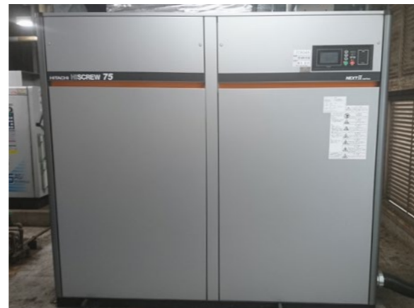
New air compressor in Factory 3
