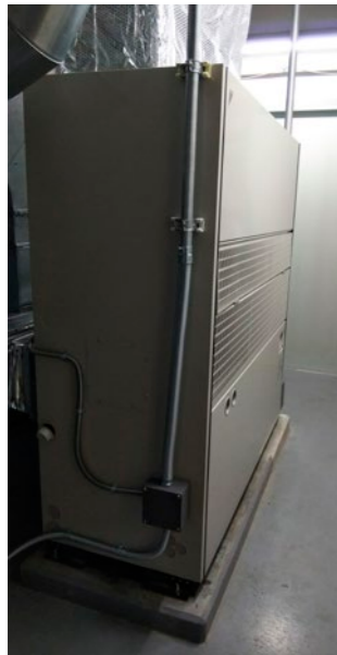
New HVAC unit for the precision measurement room
